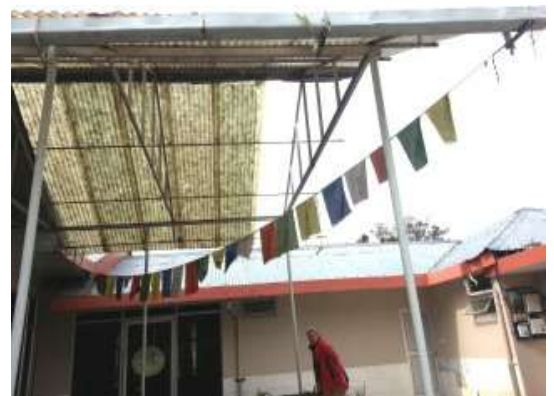
This is the current construction - a half-roof of flimsy plastic corrugated sheets
